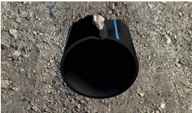
Point type damage in case of PE100 or PE80 standard pipes
